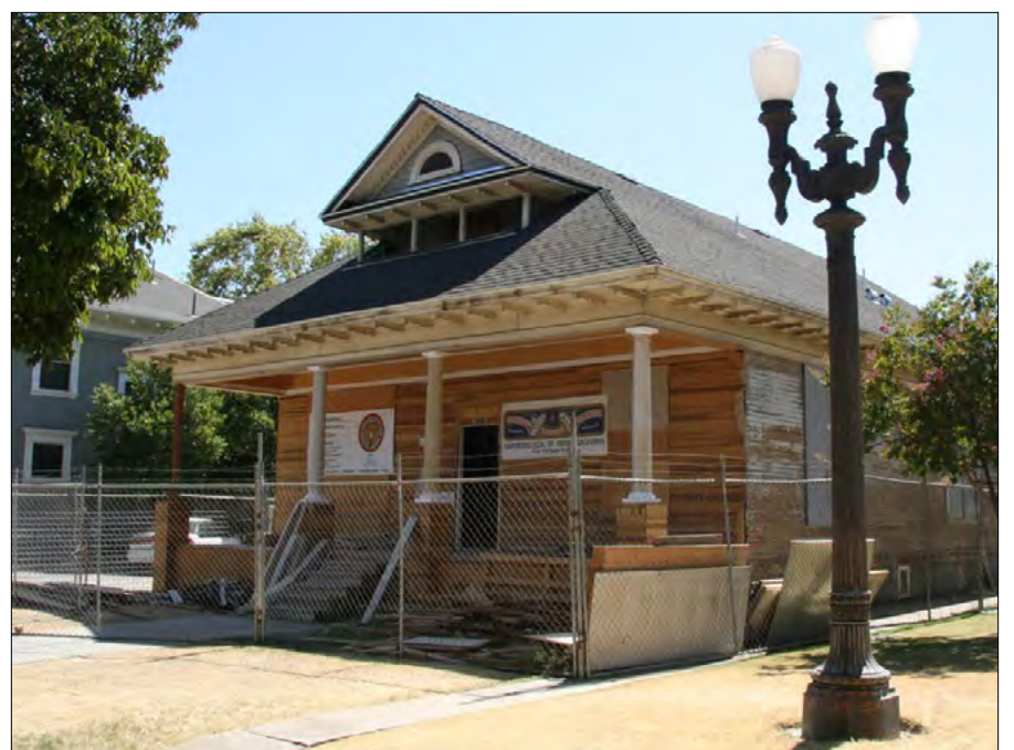
Towne Apartments (ca. 1902) have been renovated and rehabilitated in a manner that is faithful to its historic style.
